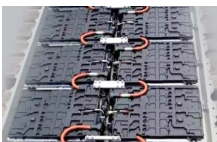
Battery charge/discharge test
